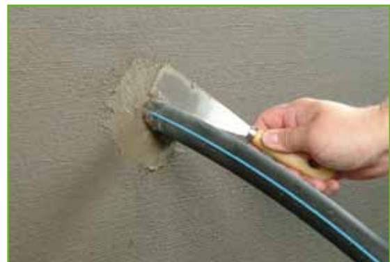
The pipe penetration is now waterproof. In order to protect the waterproofing the area around the pipe or cable is plugged with KOSTER KB-Fix 5.
