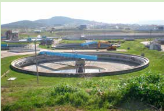
Sewage treatment plant, Istanbul, Turkey
