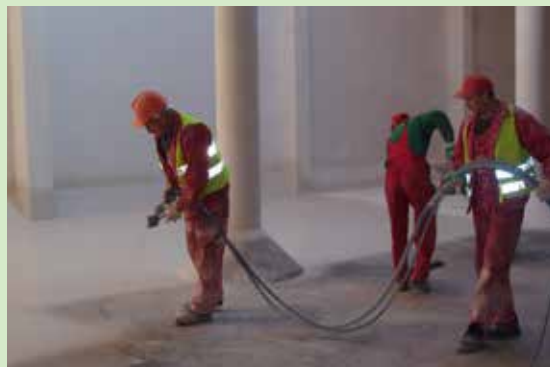
Drinking water tank, Tarnów, Poland
