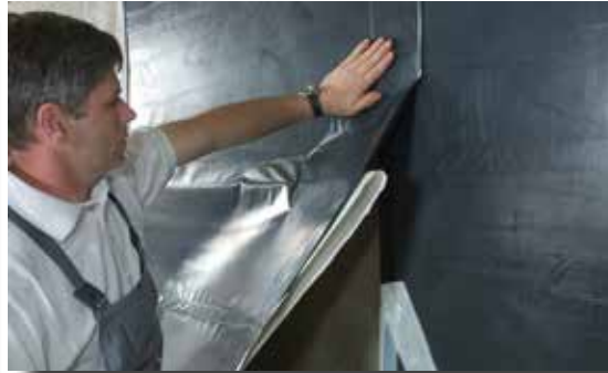
The area is waterproofed with the membrane. Membranes must overlap by approx. 4".
