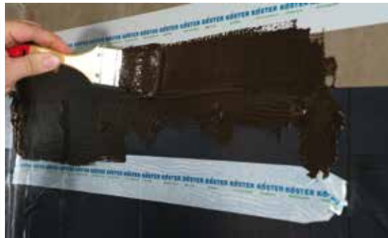
The edges of the membrane are sealed with KOSTER KBE Liquid Film.
