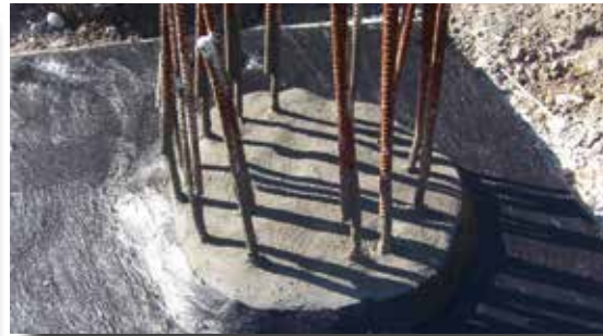
Connection of the area waterproofing (KOSTER Deuxan®) to the pile head waterproofing
